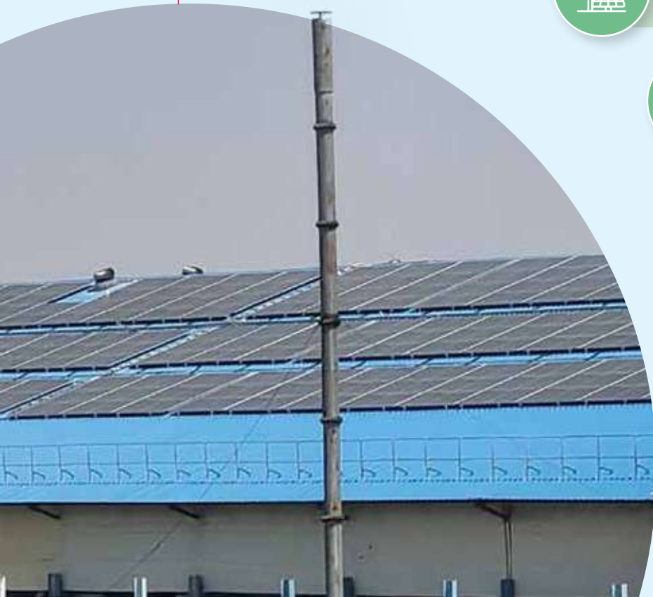
Rooftop Solar at Jainpur Plant
